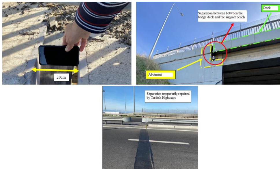
Figure 6. Deformation observed as 15-20cm separation between the bridge deck and the support bench
